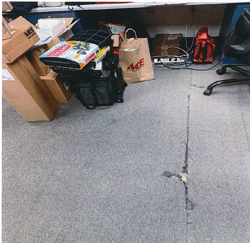
Ripped carpeting in the office
